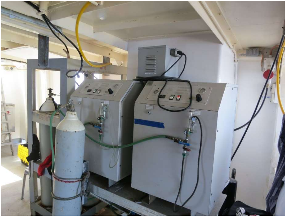
Oxygen generators & storage cylinders.
